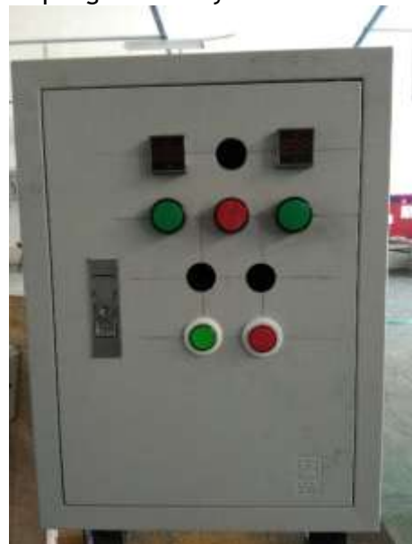
Gambar 5 Panel Kontrol PLTA PH
